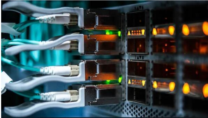
Networking (ICT) Platform
